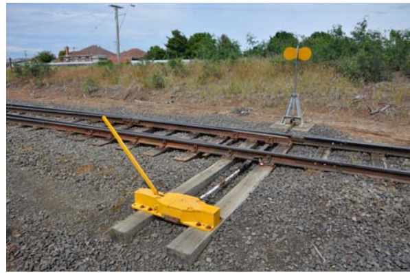
A set of points locked (see close up below)
