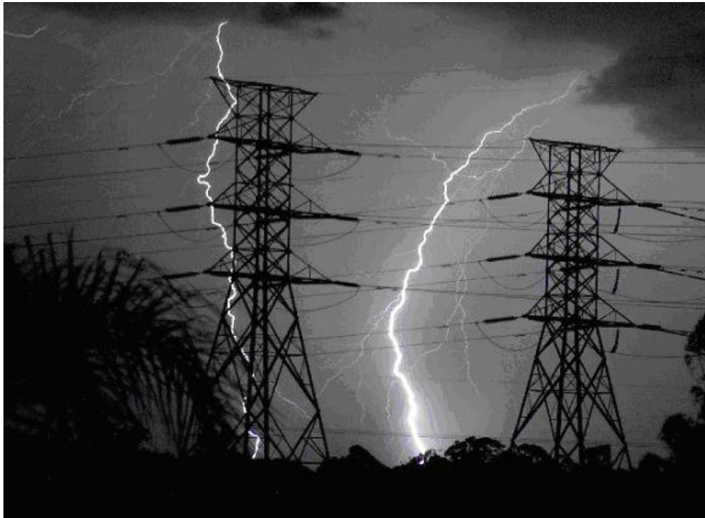
Figure 43 High voltage transmission cables in an electrical storm
