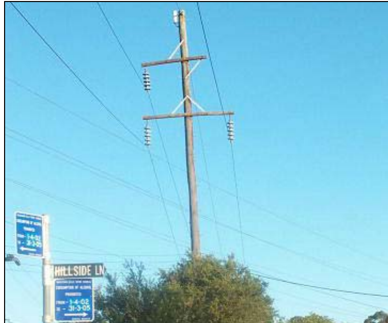
Figure 6 Sub-transmission pole line
