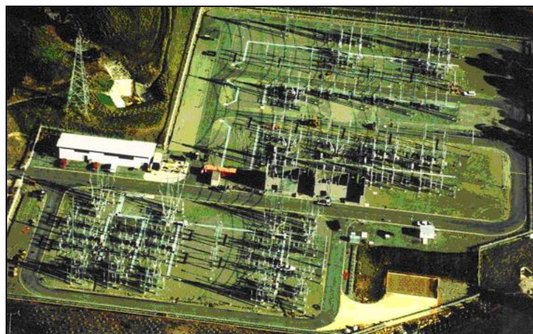
Figure 7 Bulk supply point
