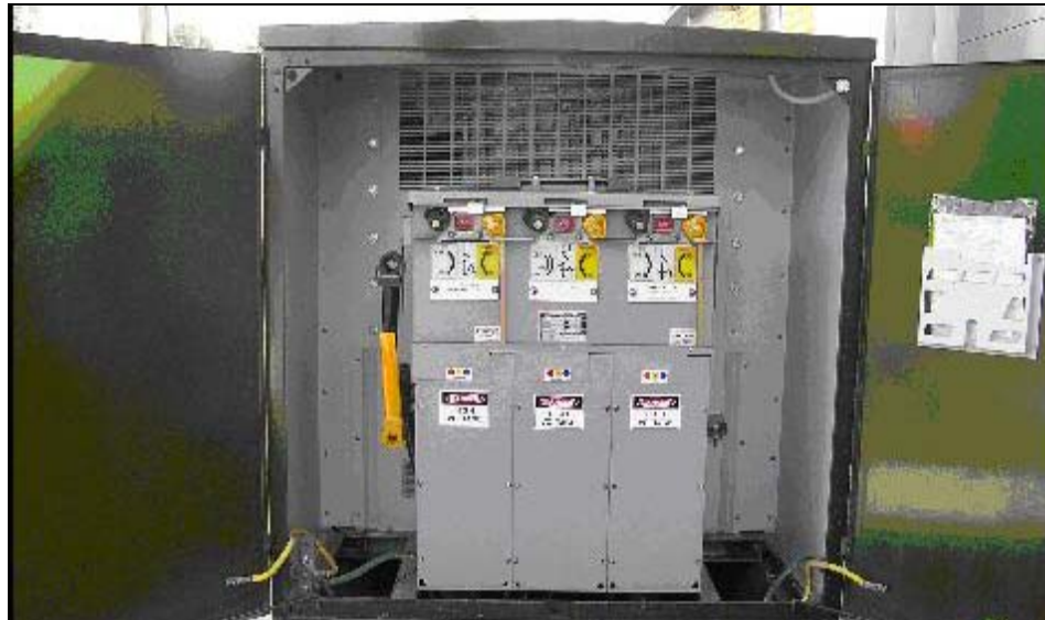
Figure 13 Kiosk—Internal view of the high voltage end
