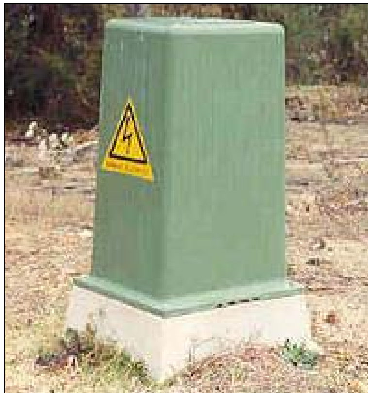
Figure 16 Underground power pillar
